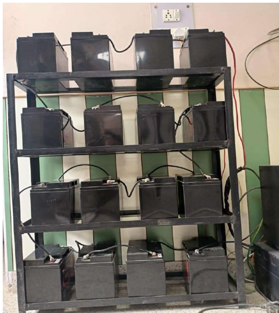
Power backup Administration Office
