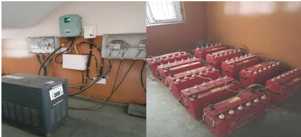
Power backup for Solar Energy
